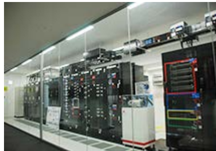
Demonstration facility electrical lab
