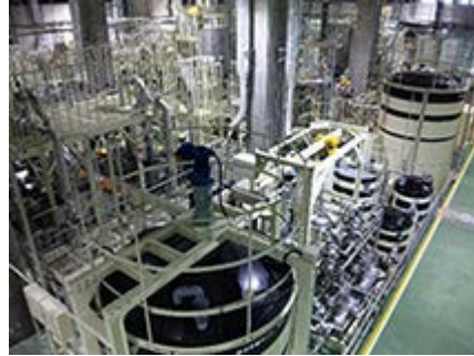
Water recycling equipment
