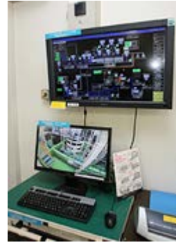
Detoxification and water recycling equipment is monitored on a 24-hour basis.
