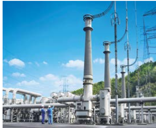
Mitsubishi Electric Transmission and Distribution Systems Center, ensuring exacting standards of quality for one of the world's most reliable power distribution systems. Its products are in use globally.
