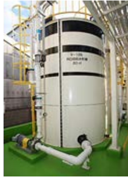
Recycled water storage tank.
