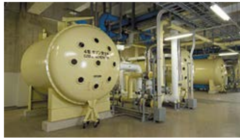
Ozone generation equipment
