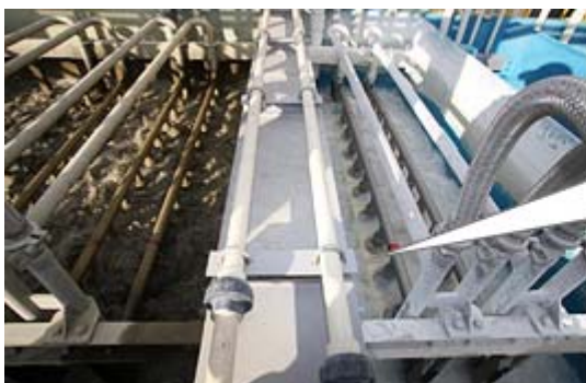
Water detoxification equipment at metal plating facility.
