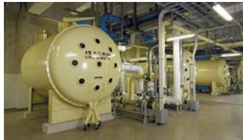
Ozone generation equipment
