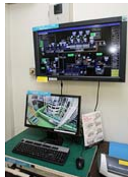
Detoxification and water recycling equipment is monitored on a 24-hour basis.
