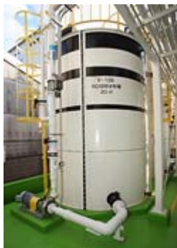
Recycled water storage tank.
