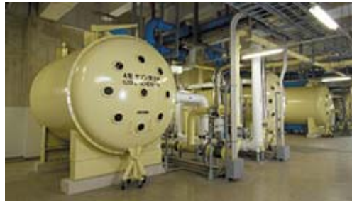
Ozone generation equipment
