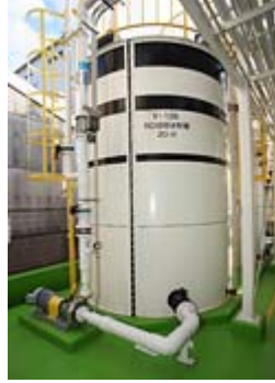
Recycled water storage tank.
