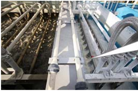
Water detoxification equipment at metal plating facility. Vat at left is for heavy metals; vat at right holds water containing fluorine.
