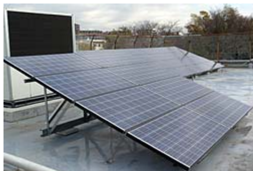
Photovoltaic panels installed on roof
