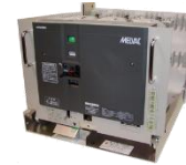
Vacuum circuit Breaker
