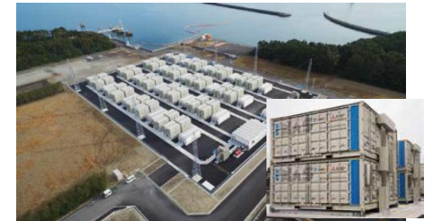
Energy storage system
